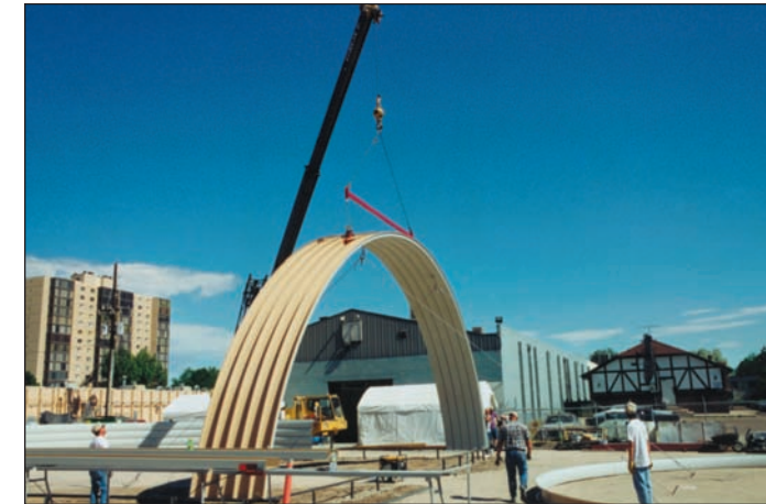
Five curved arches are seamed together on the ground, and set in place on the foundation steel.
