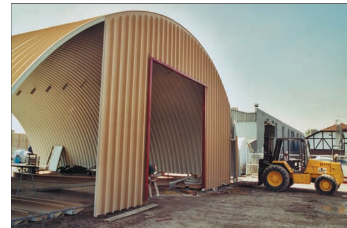
Door and window frames are installed as the end walls are being erected.
