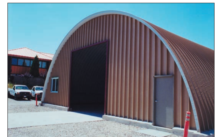
After all panels are welded or fastened to the foundation steel, the end cap is set, and concrete is poured.
