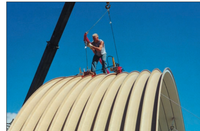
Next set of arches are nested over the first set, seamed together and welded to the foundation steel.
