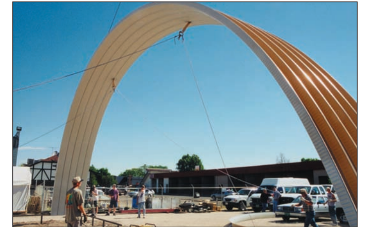
First group of arches are tied off to hanger brackets, plumbed and squared, and welded in place.
